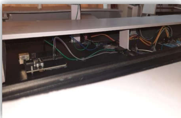
Fig:[4] connection of Arduino for an inter-platform bridge
