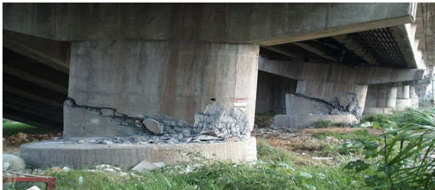
Seismic failure of bridge.
