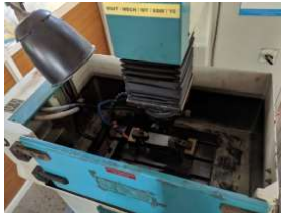
Figure 3: Dielectric Fluid Tank
